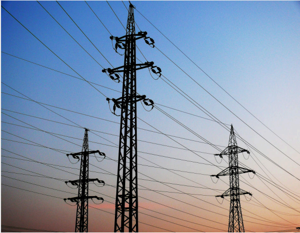
High voltage lines
